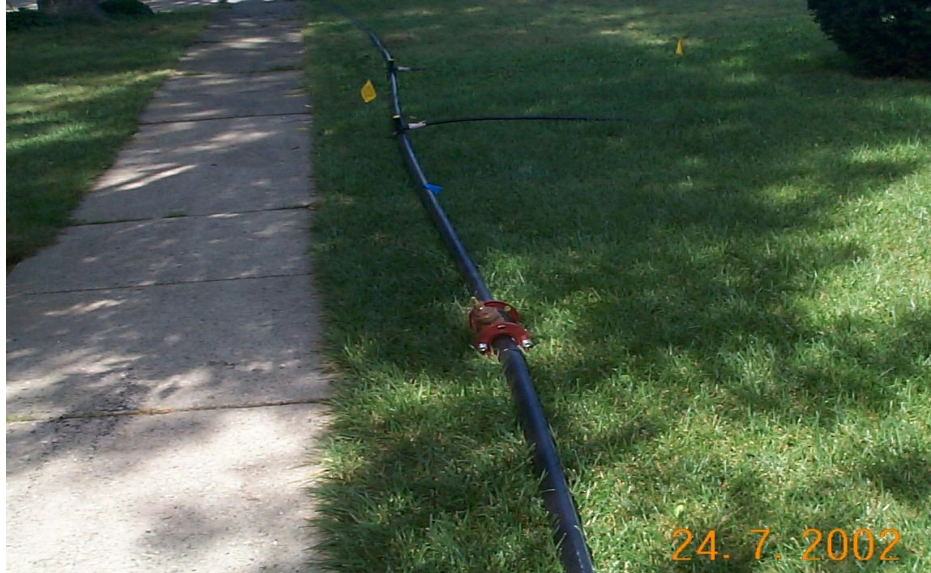
Figure 20 – 2” HDPE Temporary Water System W/ In-line Valve & Electrofuse Saddles W/ ¾” HDPE Service Lines
